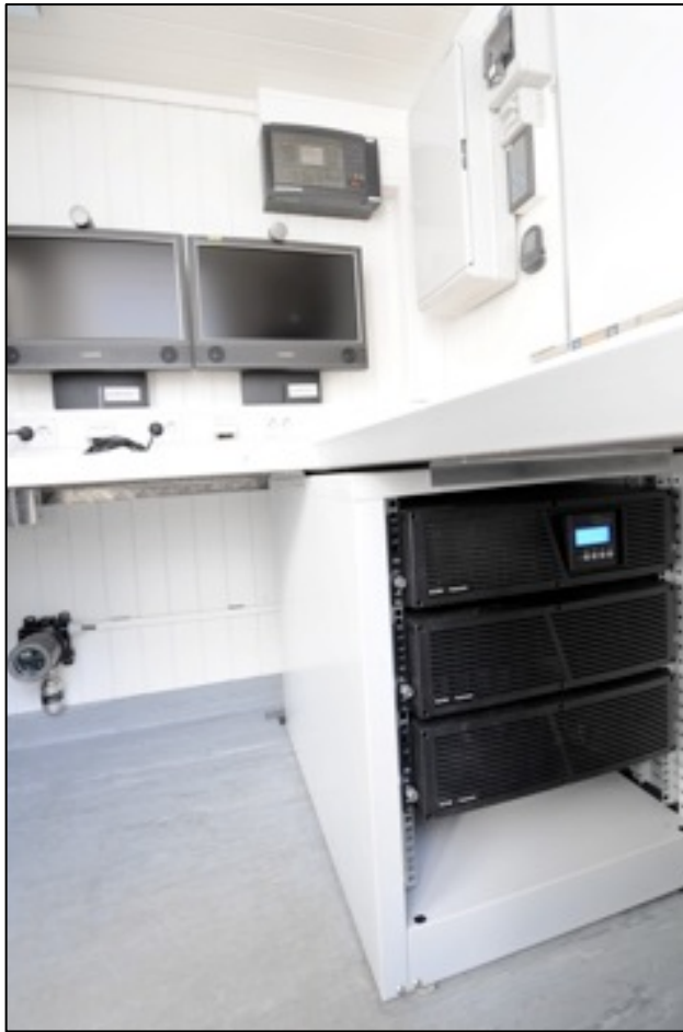
MCC UPS and Alarm panel
